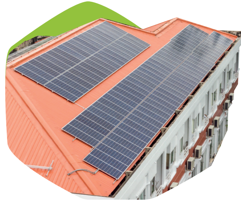
SOLAR PANEL FOR COMMERCIAL BUILDING
